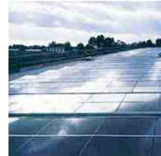
Illustration 1: Example Roof-mounted Solar Array
